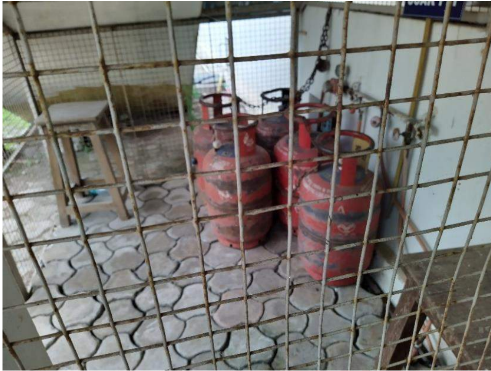
LPG cylinders placed outside the room and well protected with strong mesh.
