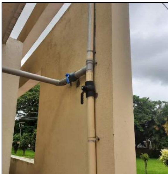
Rain water harvesting at Bagewadi College.
