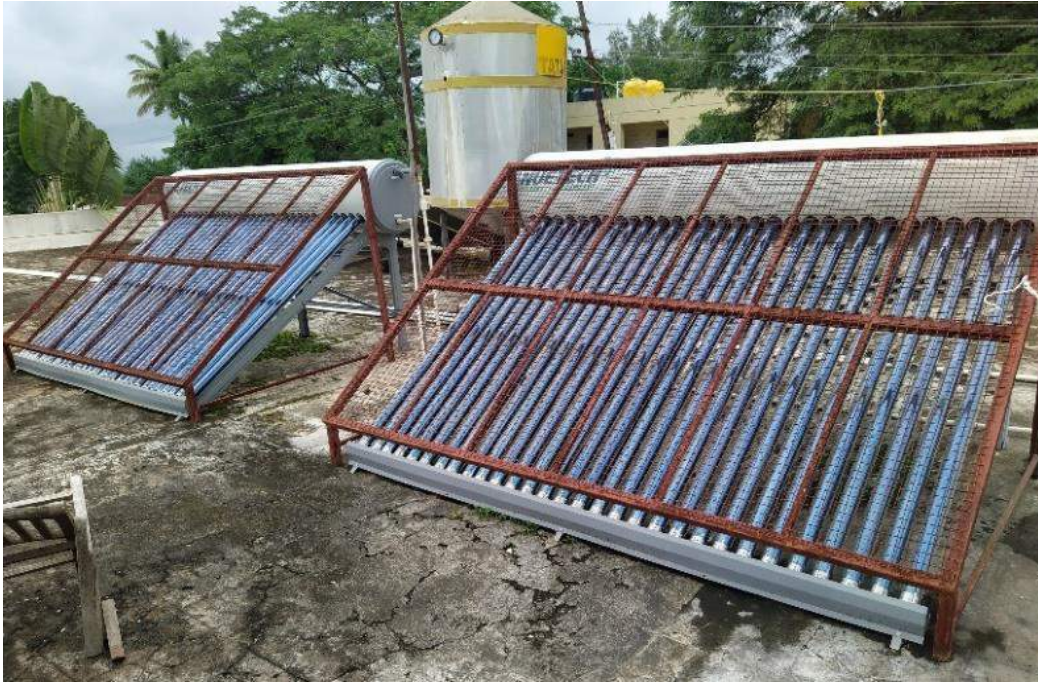
Protecting the assets and use of Renewable energy.
